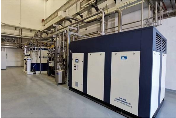
China company made 850kW@4K cryogenic plant installed in IHEP South Ligh Source test facility in Dongguan (May, 2022) (Next step is 10~18kw@4K)
