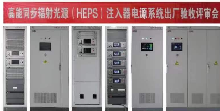
HEPS power source for magnets (June 2022)
